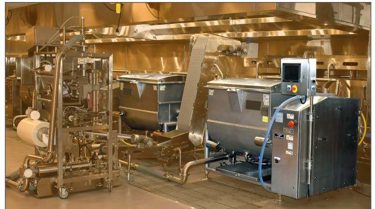
Industrial kitchen with two kettle cookers installed.
